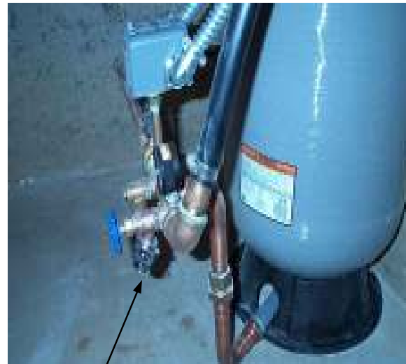
Pressure tank sampling tap
